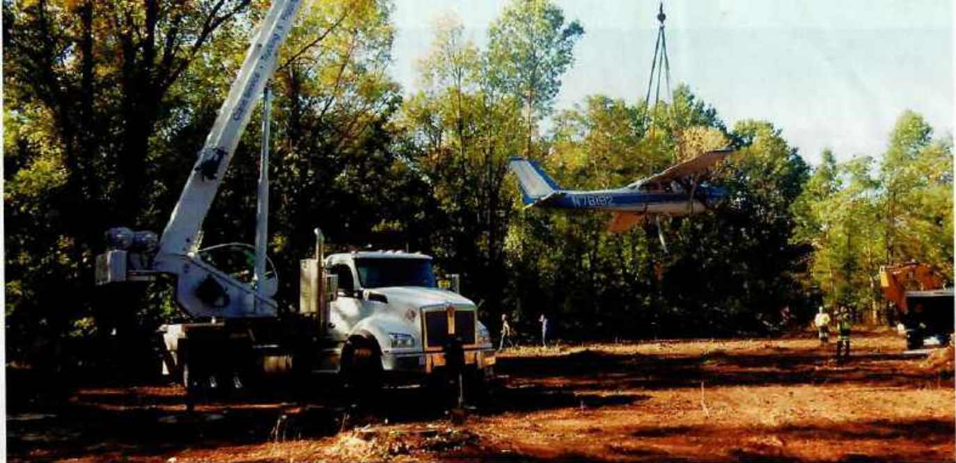
A full day of road-cutting preceded the recovery clear a path to get all the needed equipment on-scene.
